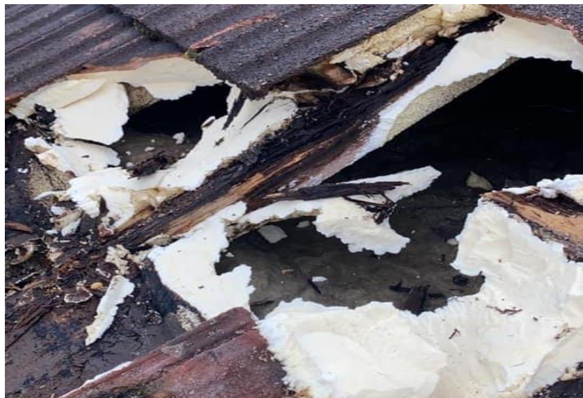
Fig 8. PU foam concealing the extent of decay in a tiled roof
