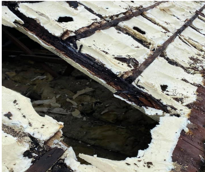
Fig 6. Closed cell foam used to stabilise a roof that has subsequently failed
