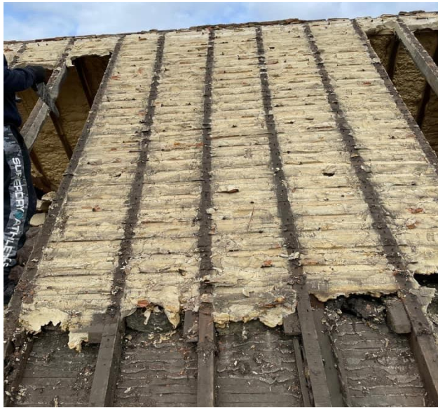
Fig 5. Closed cell PU foam applied to the extent of the available access from the void. This has left an uninsulated / bonded section of roof / ceiling in the room below. The foam has also eliminated ventilation into what should have been a cold roof void.
