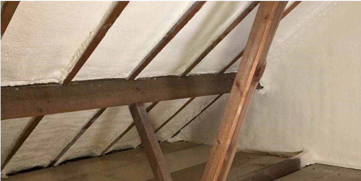
Fig 7. Closed cell PU foam applied to roof pitches and gable wall. Without detailed information from the installer, or opening up, it is not possible to assess the condition of purlin ends as they bear into the gable masonry or the wall plates or see if a breather membrane exists between the foam and roof coverings. Establishing if the void as a warm or a cold space (that should be adequately ventilated) may also be difficult here?
